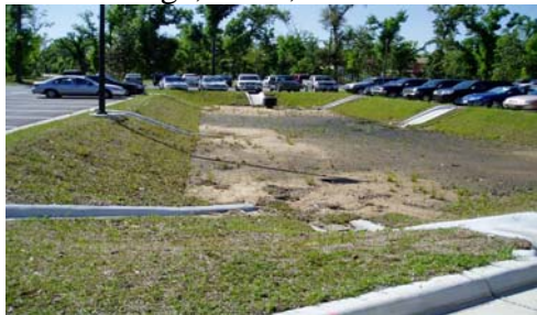
New Drainage, inlets, and retention area
