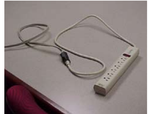
Figure 2: Mixed daisy chain—Power strip energized by an extension cord
